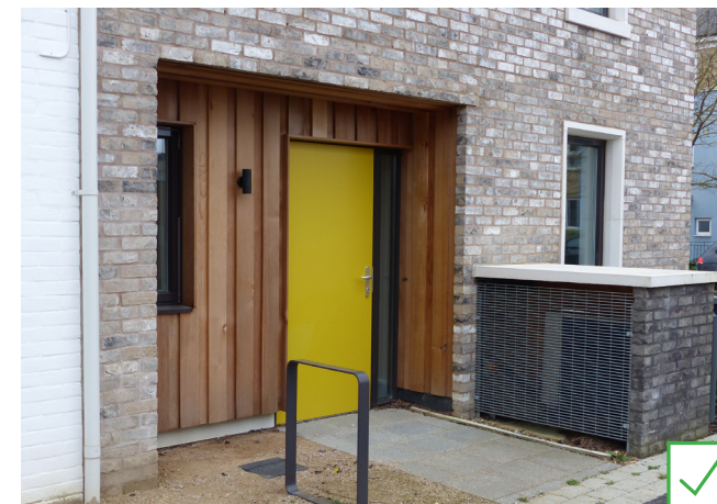
Example of a well concealed air source heat pump
